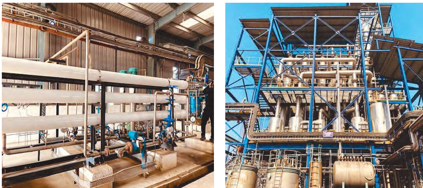
Figure 19 (Top-Left) RO based Condensate Polishing Unit; (Top-Right) Multi Effect Evaporator
