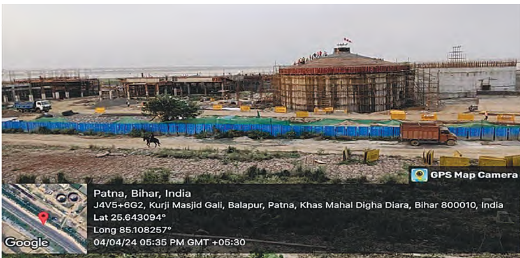
Figure 130 Digha STP and Sewerage Network 100 MLD
