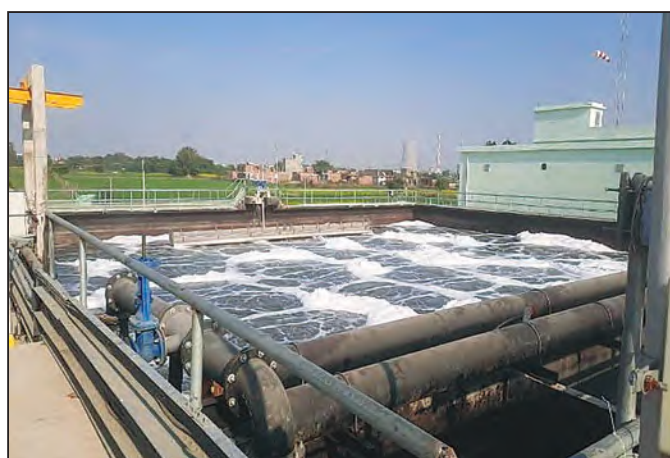
30 MLD Sewage Treatment Plant at Pankha, UP
