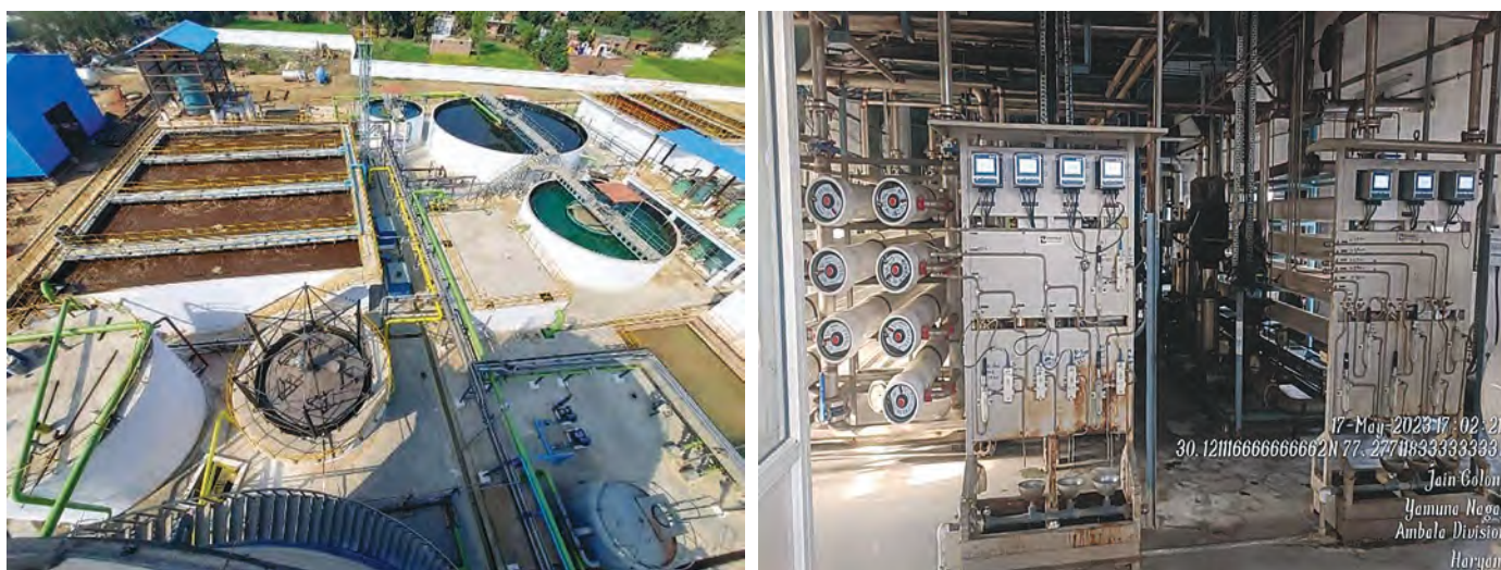
Figure 20 (L) Aerial View of ETP System at Sugar Mill and (R) Condensate Treatment Plant 4 Stage RO Unit
