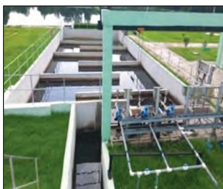
20 MLD STP at Masani
