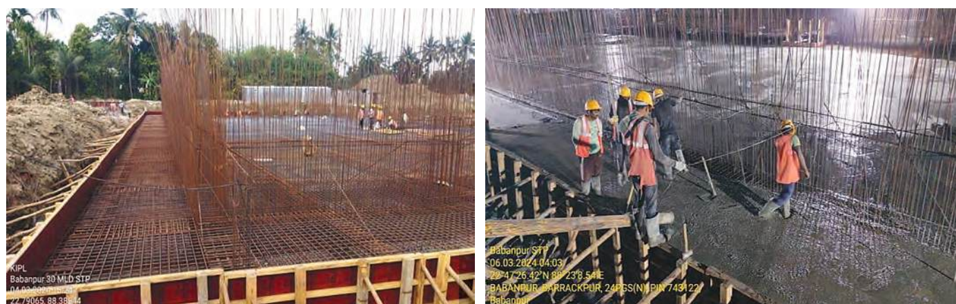
Figure 144 STP at North Barrackpore Municipality
